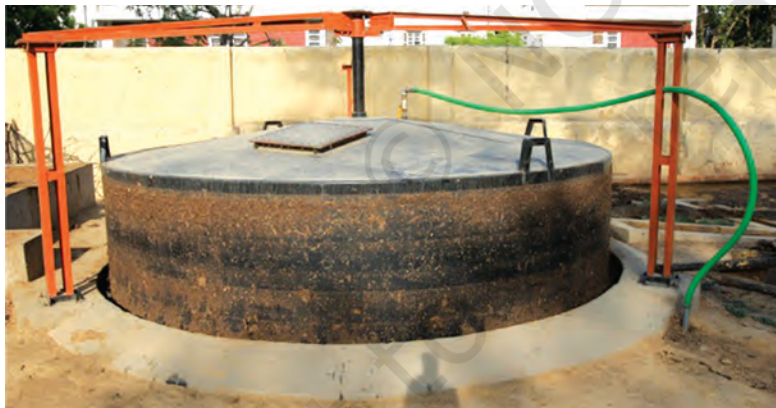
Fig. 1.15: A biogas production unit
